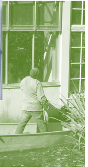
Jason Thomas repairs Conservatory windows with the help of crew member, Cholmondeley
